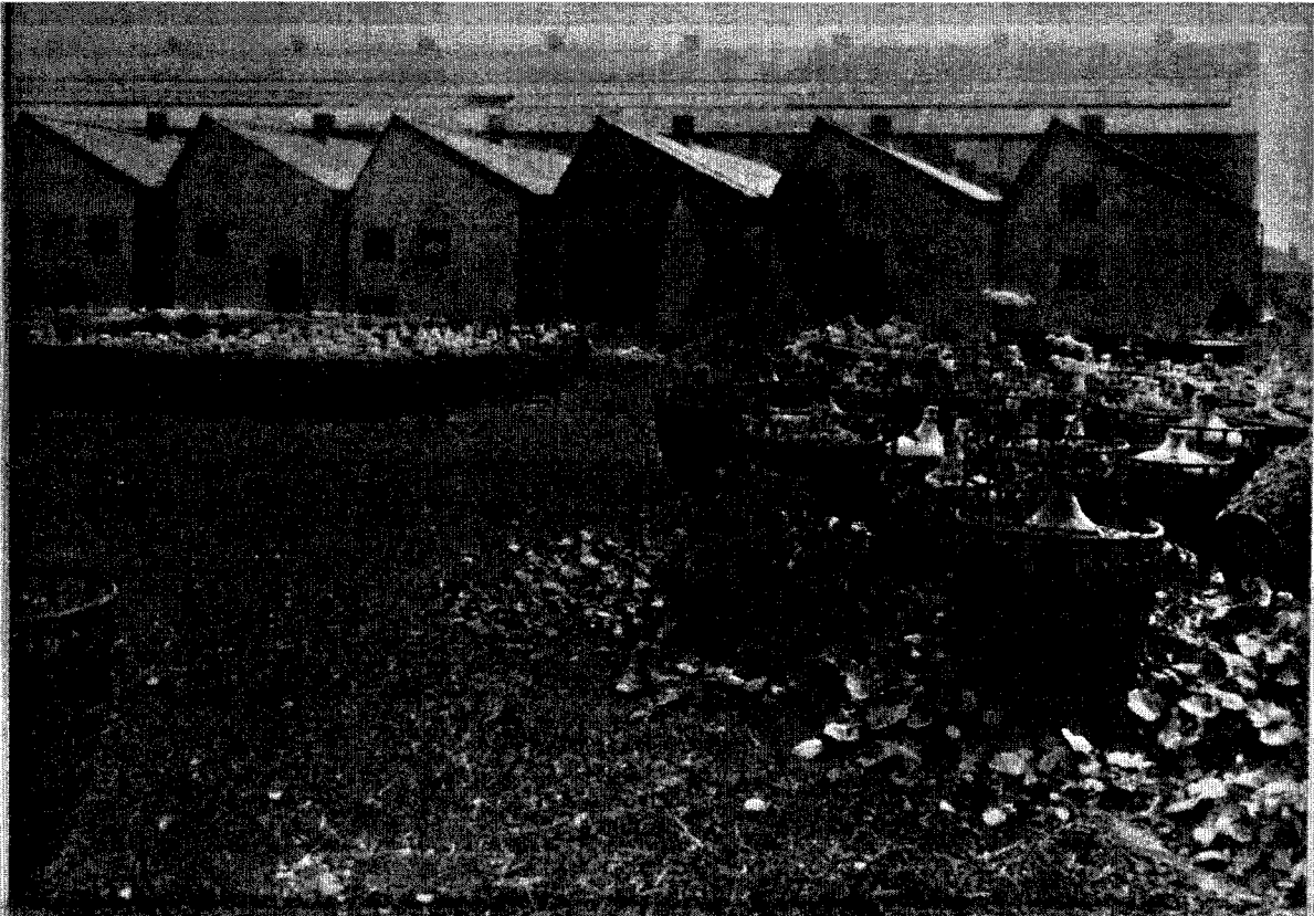
General exterior view of damage by fire to the Telephone Cable Section taken from the edge of the Cooling Pond.
